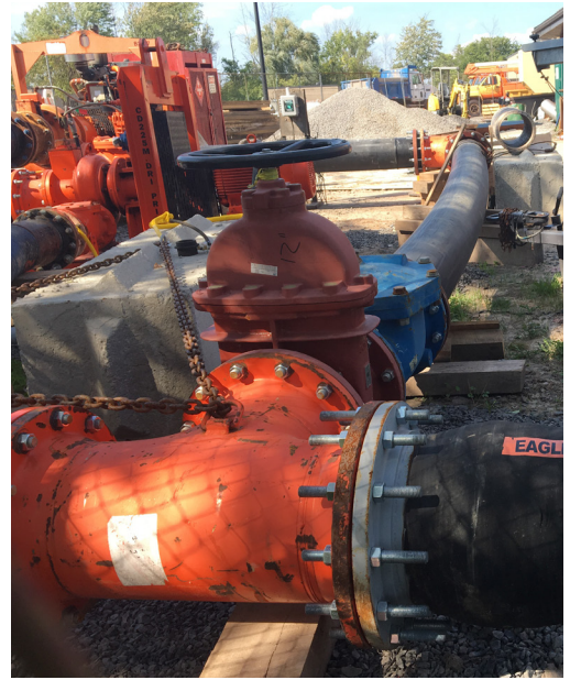
A manifold and lifting bail connects the Godwin Dri-Prime CD225M 8-inch electric pump with the Flygt N 3301 electric submersible pump (not visible).
