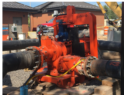
A close-up view of the 12MGD bypass system in Monroe County, New York. The solution was comprised of Godwin and Flygt brand equipment, including the Godwin Dri-Prime CD225M 8-inch electric pump.
