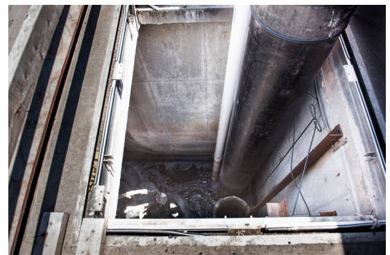
The pump station wet well. Our Flygt submersible pump is located to the left inside the pit.
