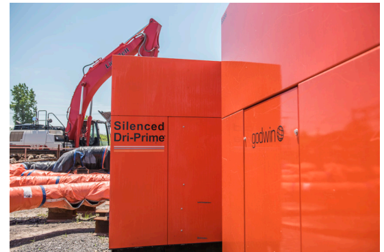
Two of three Godwin CD300s Dri-Prime diesel pumps onsite, which are the workhorses of the system.
