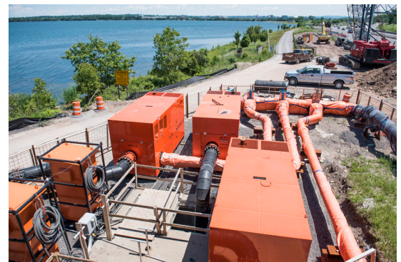
The complete Xylem solution - a 30MGD bypass system - is captured here with the city of Syracuse, New York, in the background. The solution comprises Godwin and Flygt brand equipment, including custom pipework.
