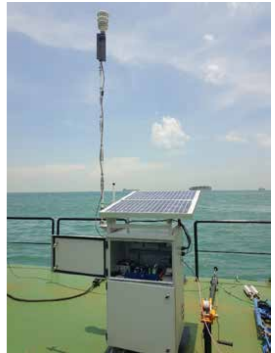
Figure 3: Datalogger, meteorological and current sensors are powered by solar power.
