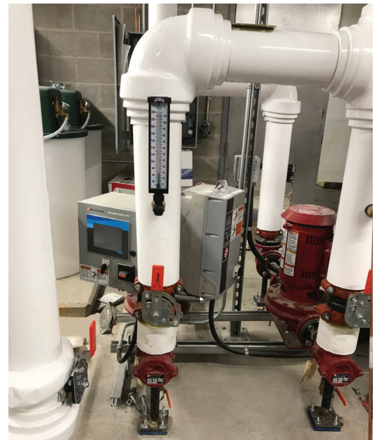
Installation with Series e-80 pump, Technologic IPC variable frequency drive and Technologic PPS controller
