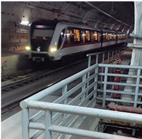
Pump installation pit at the foot of the track.
