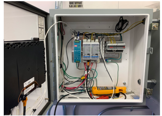
Sunriver upgraded from the trial DP control system to the full XPC Control Logic system in 2020.
