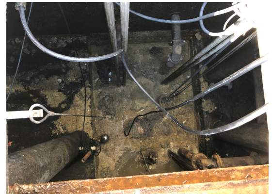
Before installing the Concertor pumps, Lift Station 3 experienced constant blockages.
