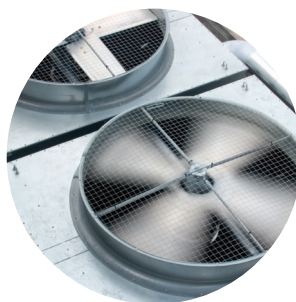
Heating, ventilation and air-conditioning (HVAC)
