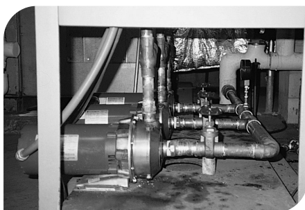
Pressure booster system
