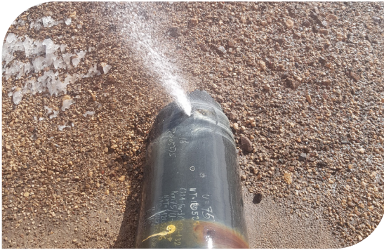
Collect data on leak location, magnitude, and type (joint, barrel, or feature leaks)
