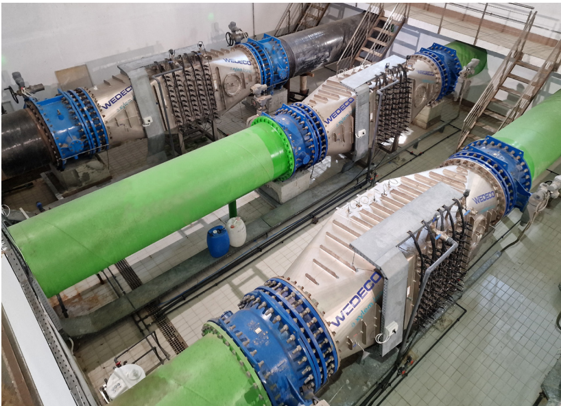
Reactors in operation.
