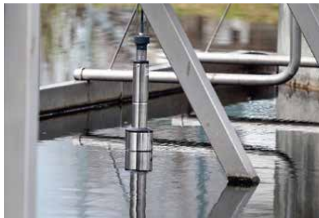
Fig. 2, Typical location of the IFL 700 IQ on a scraper bridge in the secondary clarifier.
