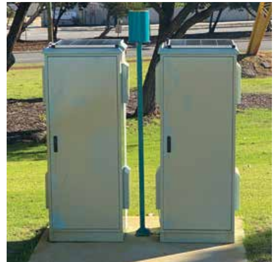
Figure 3 Instrument Enclosures and Rain Gauge
