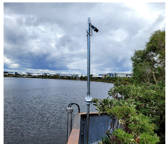
Figure 3. Solar Water Quality Monitoring Station
