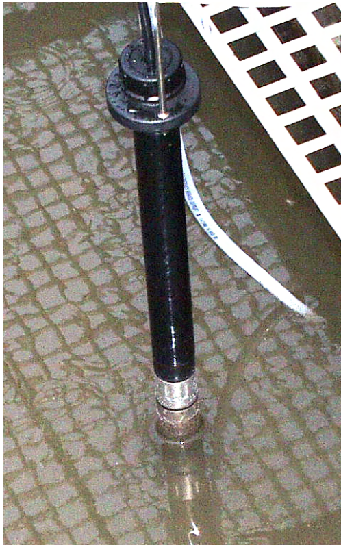
Fig 12 VARiON Plus 700 IQ in the activated sludge basin
