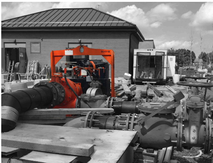
A temporary bypass system, which included a Godwin Dri-Prime CD300M 12-inch diesel pump and Godwin Dri-Prime CD225M 8-inch electric pump, operated continuously for three months during equipment upgrades at the John Street lift station in Monroe County, New York.
