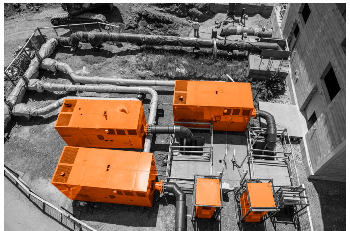
A combination of diesel pumps and electric submersible pumps allowed the temporary bypass project in Onondaga County, New York, to operate at maximum efficiency, offering a flexible solution for fluctuating wastewater flow levels.
