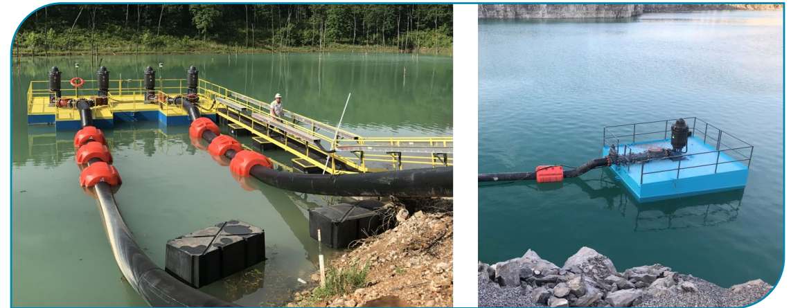
Turbine Pumps on pontoons
