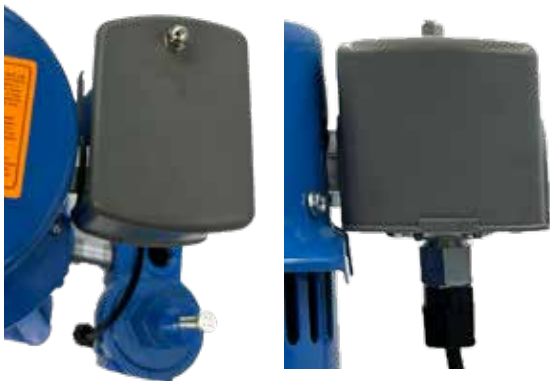
Grey brandless motor controller with no warning sticker
