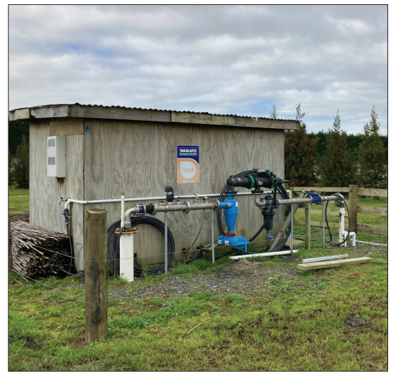
The pump shed where the wall mounted HYDROVAR variable speed drive is located to control the Lowara Z646 11-6 pump which supplies water for the farm's varying irrigation demands.
