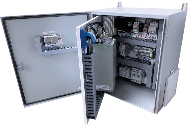
CAPAC system power supply controller (PSC)
