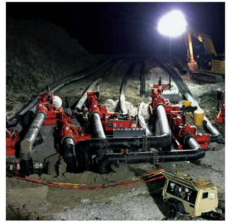
Xylem and the contractor teams worked around the clock to get the first pumps in place in six days.
