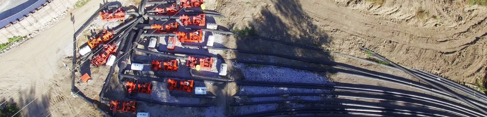
Aerial shot of the suction pit, with the discharge tubes running off into the lower right corner of the image. To the upper left of the suction pit is the retaining wall that was installed adjacent to the parking lot.
