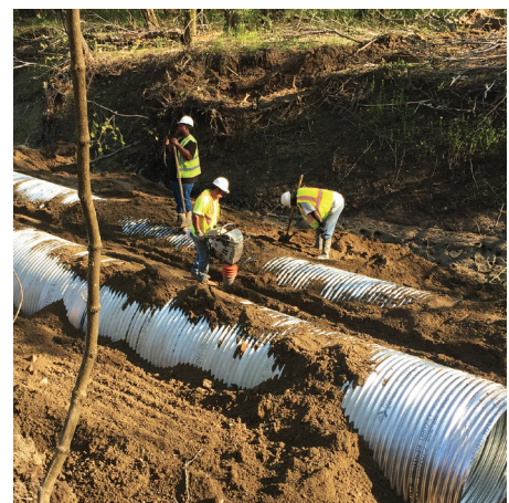
A culvert was put in place along 100 feet of the bypass line where the bypass crossed Cypress Creek.
