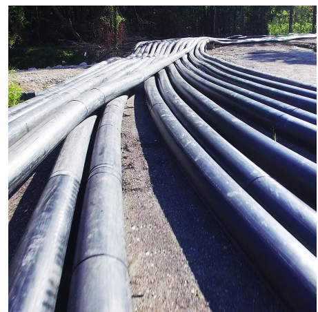
A 40-foot wide right-of-way was constructed to handle the nearly six miles of pipe mobilized for the bypass. This section shows pipes heading towards the discharge structure 2,400 feet away.
