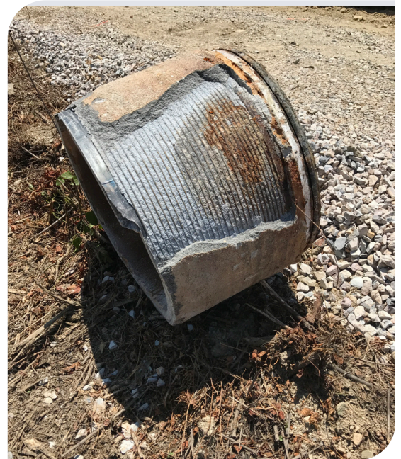
Hot Springs field technicians quickly located an issue with this 24-inch prestressed concrete pressure pipe thanks to advanced leak detection technology.
