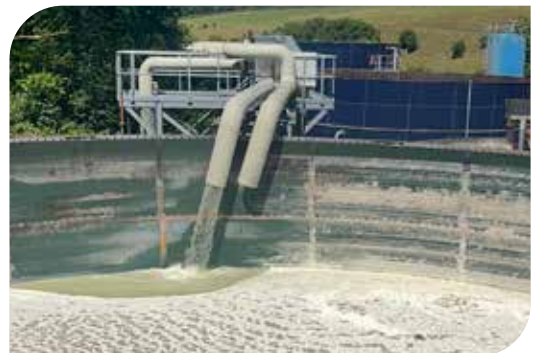
Dairygold anaerobic digestion wastewater treatment
