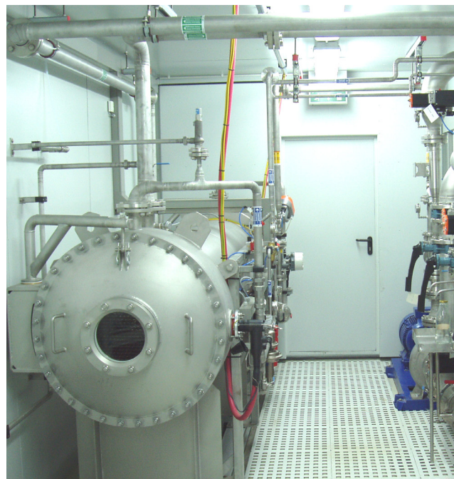
WEDECO Ozone generator and injection system
