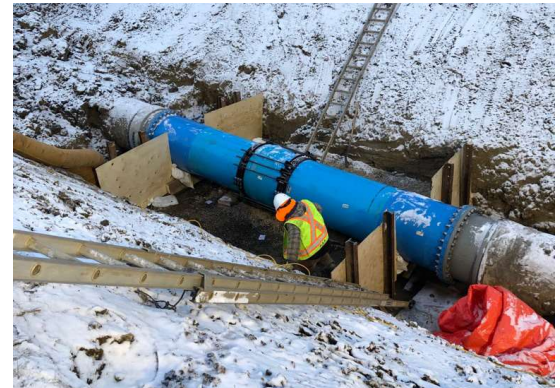
EPCOR conducted an emergency repair on this high-risk pipe in December 2019. Inspections identified a leak on the pipe barrel and broken wire wraps.
