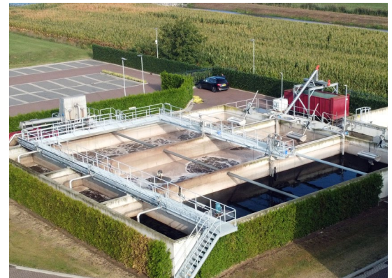
Prochamp's green treatment plant with SBR technology
