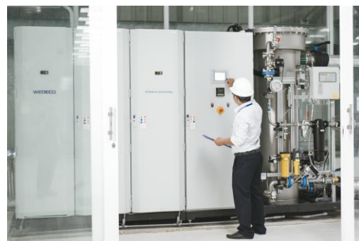
Xylem Wedeco SMOevo ozone system, Vietnam's first ozone system
