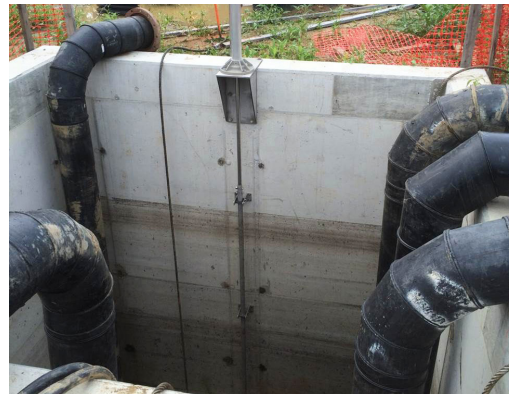
High-density polyethylene pipe exiting the wet well.
