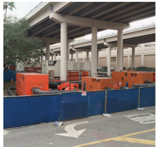
The bypass was under an expressway in downtown Tampa, which made maneuverability and equipment placement a challenge, with one lane open for traffic.
