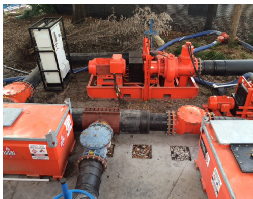
The fuel cubes, lower right and left, were used as part of the back-up redundancy of the system for the Godwin diesel-driven pumps.
