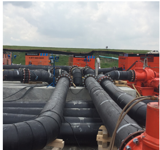
HDPE pipes running from the Godwin Dri-Prime pumps to the splitting chamber for Phase III of the bypass.
