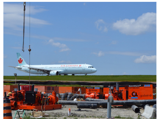
A short distance from the taxiway, pumps and piping were placed by crane at the job site.
