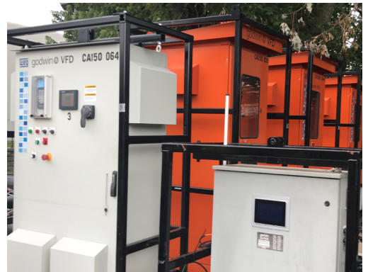
Four variable frequency drives helped maintain operation and efficiency throughout the bypass project. A Godwin Advanced RMC panel (right) provided remote monitoring capabilities, alerting crew members to potential pump issues via any smart device.
