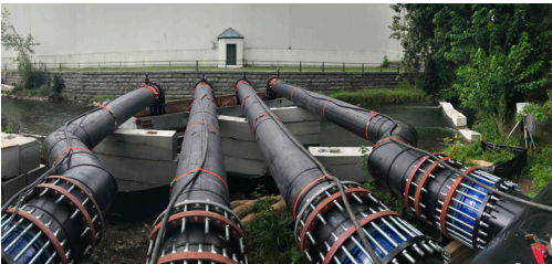
Diverting waterway flow through bypass piping enabled the dewatering of the Owasco Outlet for excavation and remediation. The bypass required four lengths of 30-inch HDPE pipe to handle the flow requirements.
