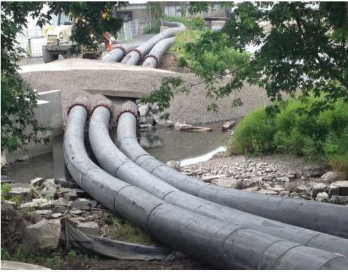
The temporary bypass setup, which operated in stages over a three-year period, employed 7,500 feet of 30-inch HDPE pipe.
