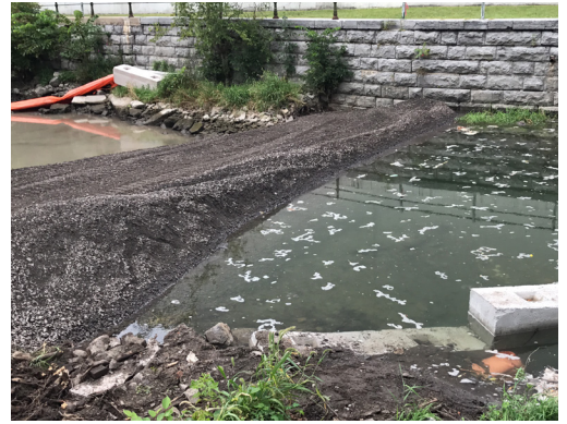
To contain the threat to wildlife during the soil remediation project, the stream bed was dried out in 1,000-foot increments, with the bypass system essentially creating two manmade dams - one upside of the stream and one downside.
