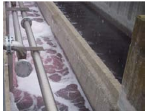
Ozone for decolouration and tensides reduction at RANICA WWTP (Bergamo), Italy
