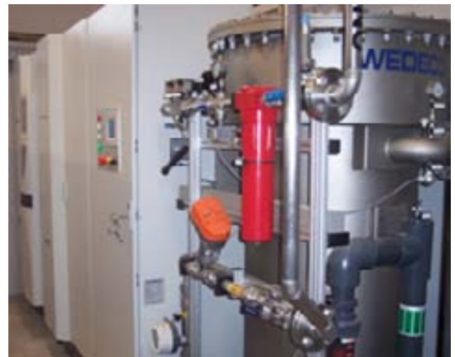
The ozone plant has been designed for a maximum ozone production capacity of 28 kg/h at 7 wt % concentration, from oxygen (pipeline), supplied by SIAD (PRAXAIR GROUP)
