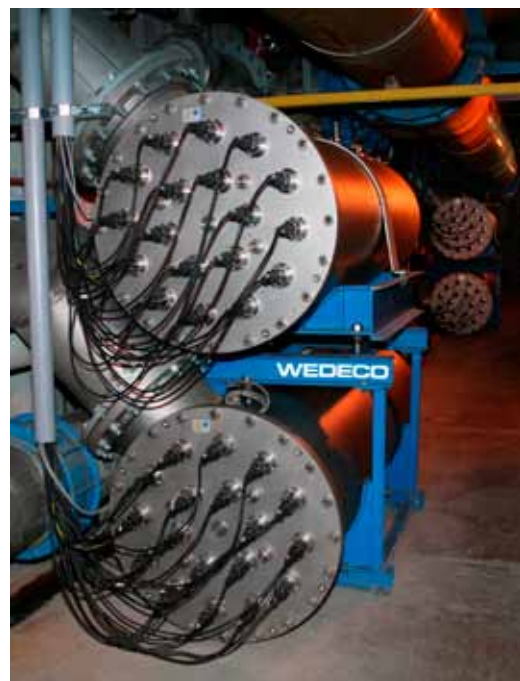
Nine ultraviolet reactors installed offering remarkable disinfection performance.
