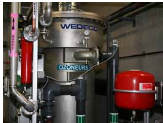
Organics and polymers broken down by two SMO700 Ozone generators.
