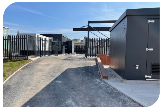
Don Street Pumping Station
