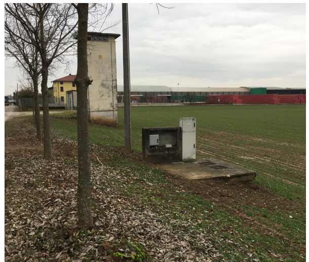
The Via Visan Malo pumping station, Marano Vicentino, Italy
