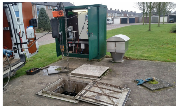
The Platenmakerstraat pumping station, Overbetuwe, Netherlands
