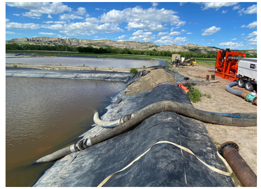
The Godwin HL270M pumped water from settling ponds to a frac pond through a seven-mile-long steel pipeline, and saved the customer 15-20% in diesel costs.
