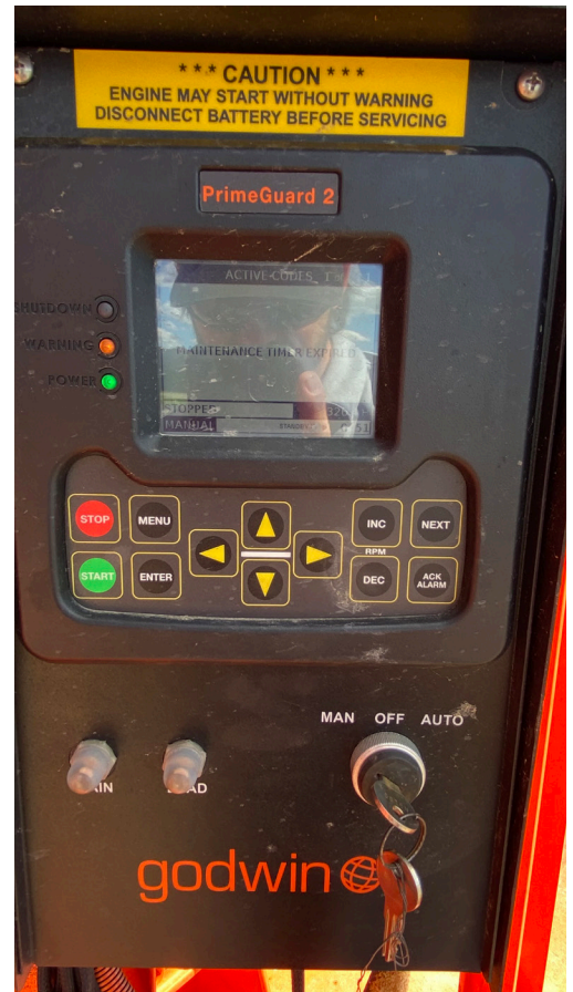
The pump's Godwin PrimeGuard 2 controller is fitted with Field Smart Technology - an advanced telemetry and cloud-based monitoring and control system which automatically alerts operators about any issue with the potential to develop into a problem. This enables operators to focus on other tasks without constantly worrying about pump performance.
