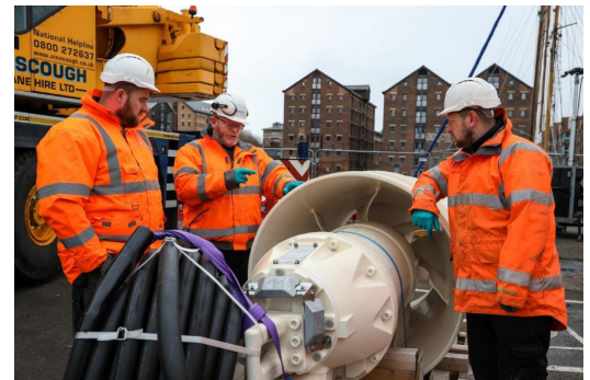
Figure 1. Engineers working with the Canal & River Trust on the installation of the new pumps in Gloucester Docks.
