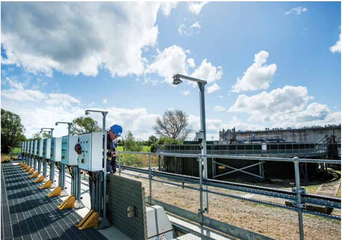
Wedeco Duron UV installation in Chichester, UK.
