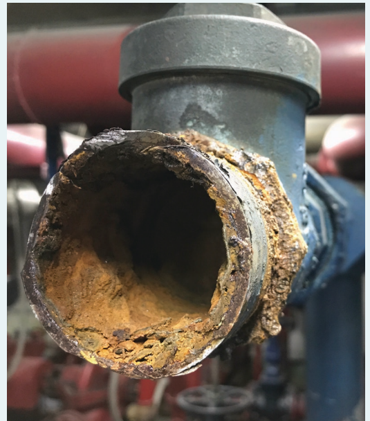
Corrosion in an iron pipe showing many areas where microbes could establish themselves
