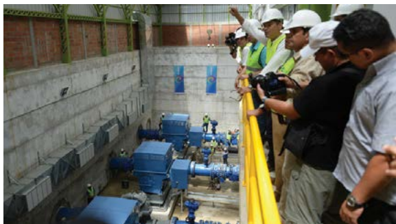
Crews look below to the newly installed Flygt pumps for the Transvase Chóngon-San Vicente project.
