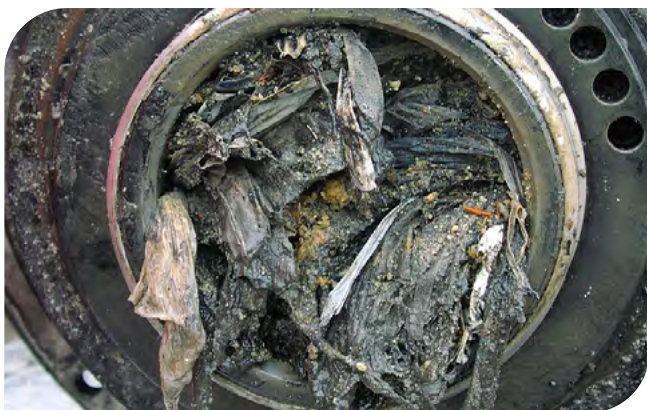
Figure 1: A fully clogged pump (pictured) is easy to detect, while a partially clogged pump is rarely detected when a pump is inspected.
