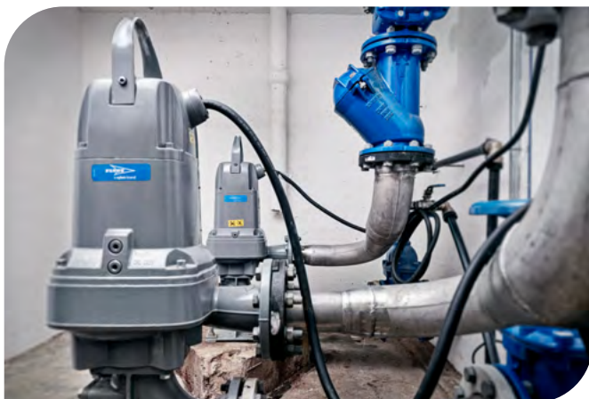
Flygt Concertor 6020 pumps, featuring Adaptive N hydraulics, in a municipal wastewater pump station
