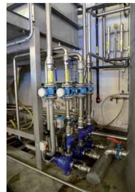
The ozone treatment plant designed by HSE obviates the necessity of weekly emptying of the washing and processing equipment
